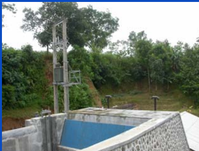
TRASH RACK Manual-Automatic Cleaning
