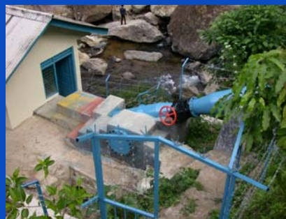
Cisanggiri, Garut, Jabar X-flow T-14, ELC-Test Plant-90 kW 2002
