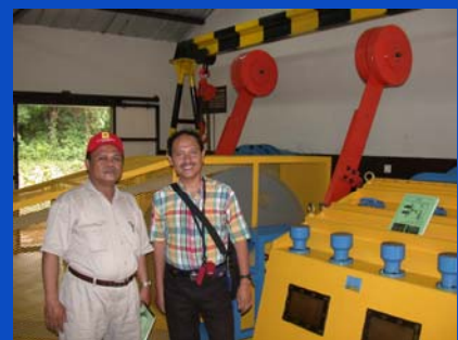
Melong, Subang, Jabar X-flow T-15 D500, ELC-100 kW-Grid PLN 2005
