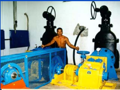
The First T-14 D300 100 kW Bili-Bili, 1999 Followed by Dewata 120 kW (2002)
