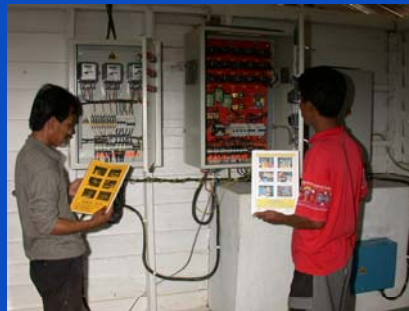
Induction Generator Controller PLTMH Cipaleubuh, Jawa Barat IGC HeksaHydro – 15 kW
