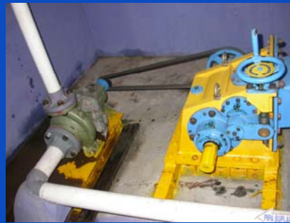
Cineang, Garut, Jabar X-flow T-14, Centrifugal Pump-2 kW 2004
