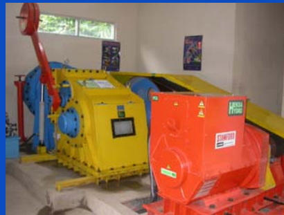
Lantan, Lombok, NTB X-flow T-15 D500, ELC-100 kW-Grid PLN 2006
