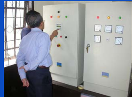
ELC-SINKRO HeksaHydro PLTMH Melong, Jawa Barat Grid Connected -100 kW
