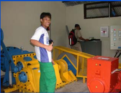
Santong, Lombok, NTB X-flow T-14, ELC-35 kW-Grid PLN 2004
