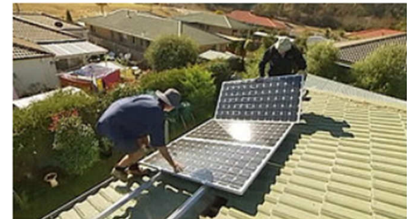
Up to 2,000 homes could be at risk of electrical fires from poorly installed roof-top solar panels (ABC News, file photo)
