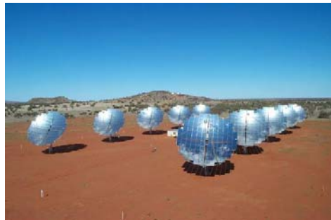
Solar Systems Pty Ltd: 220 kW PV Concentrator power plant at the Pitjantjara lands
