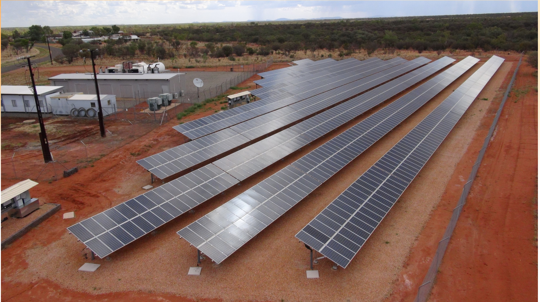
Ti Tree power station
